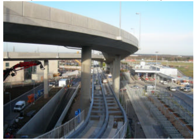
Double-track ULTra guideway threads its way under the roadway as it approaches Terminal 5
